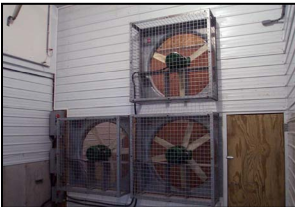
Figure 25. Modern potato storage facility with axial flow fans used to move air from the fan room to the lateral distribution ducts to maintain a constant temperature of the potato tubers.
